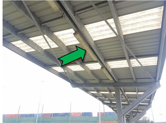
Photo 2. Exterior, throughout, double tubed fluorescent light fitting – suspected non PCB-containing capacitors.
